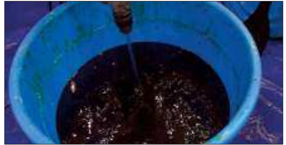
29. After 24, you can use electric drill for mixing. Do not use machine before that stage because it is dangerous.
